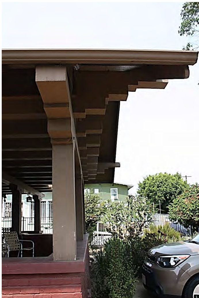
Detail: Front porch, north facing profile. Note faux pegs near the top of each box beam. Faux peg detail repeated in garage construction.
