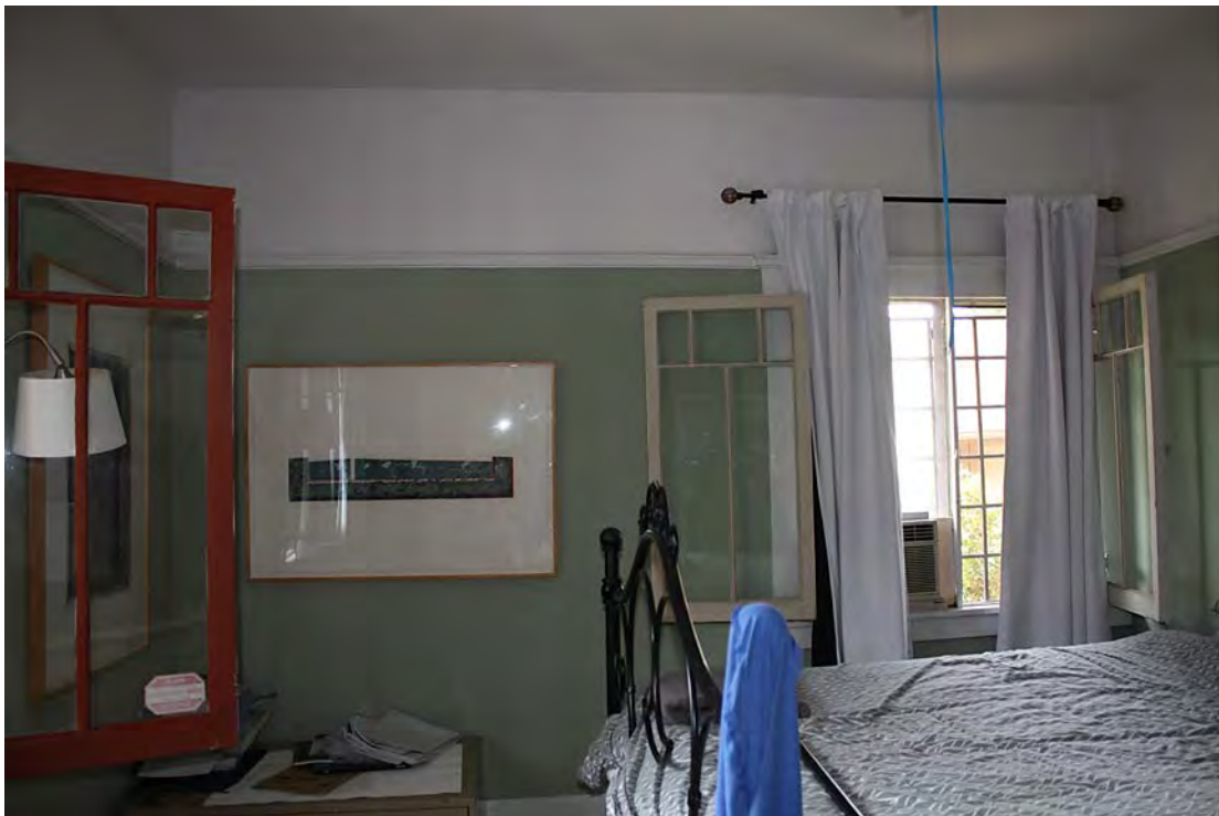
Southwest bedroom: Open one of pair of three-over-two casement windows at south wall; west wall open paired casement windows; northwest corner; picture rail around room, view west.
