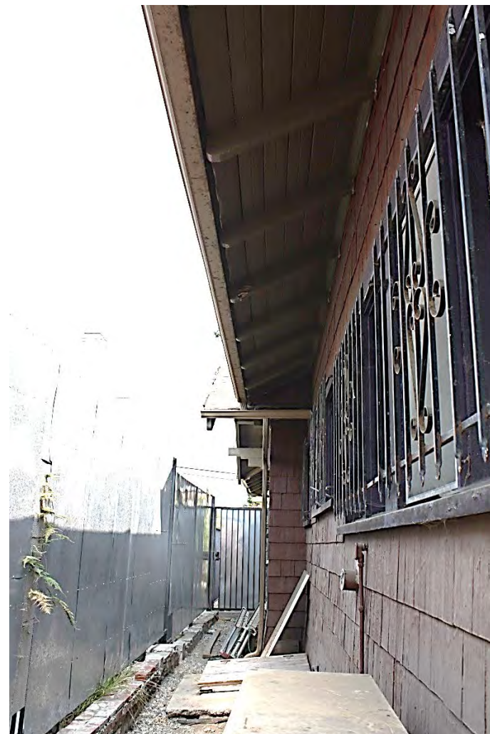
North elevation: Showing different under the eaves treatment for protruding gabled eaves, photograph at left, and main gable eaves, here. Single bulkhead door to cellar, protruding north gable area, north path with added pedestrian gate, view east.
